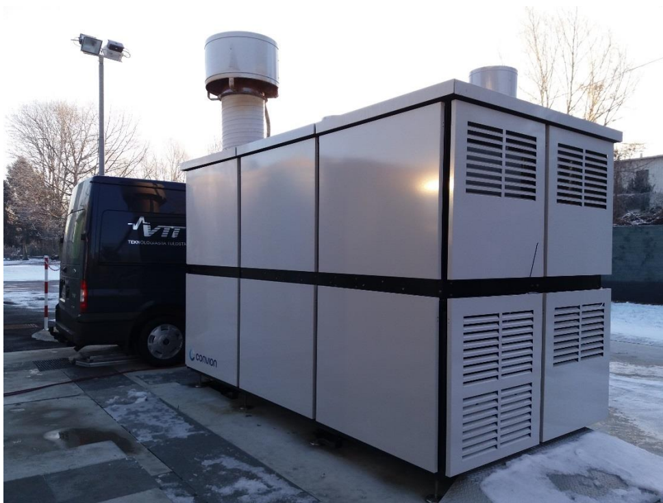
Figure 2. Setting up emission measurements. Convion C50 system in the front with VTT van with all the emission measurement equipment behind it.
